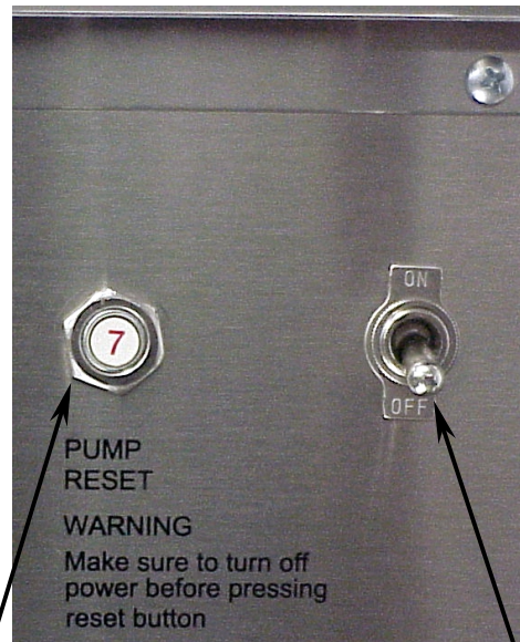
7-Amp circuit breaker
